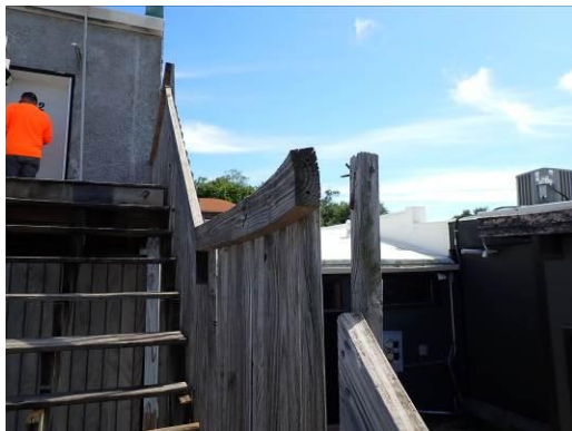
31, 32. Unsafe rail, unsafe treads
